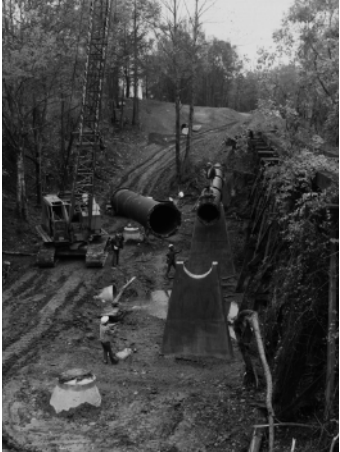
Because of ductile iron's great beam strength and durability, it is ideally suited for challenging applications such as this pipe-on-supports installation.
